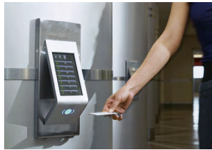
Access Controlled Elevators
